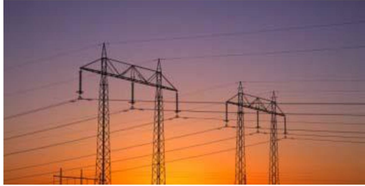
Fig.1 Shows Over headed Transmission line
