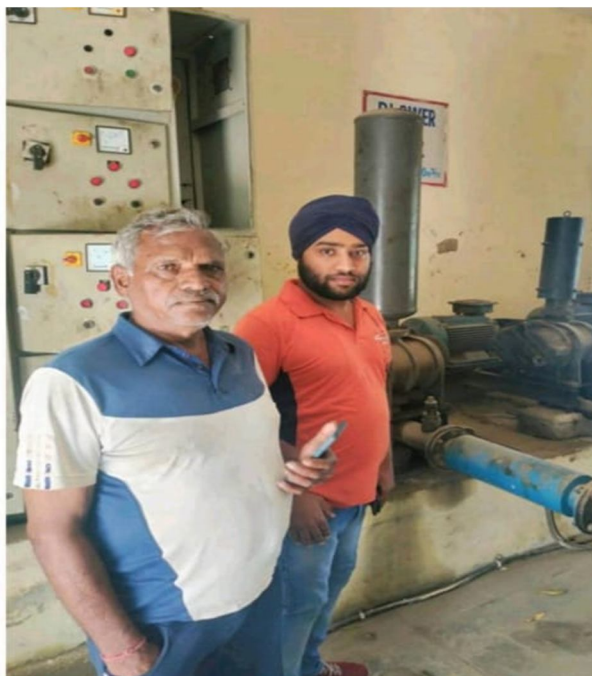
Figure 4: Aeration Unit At PHED DEVINAGAR AMBALA CITY
