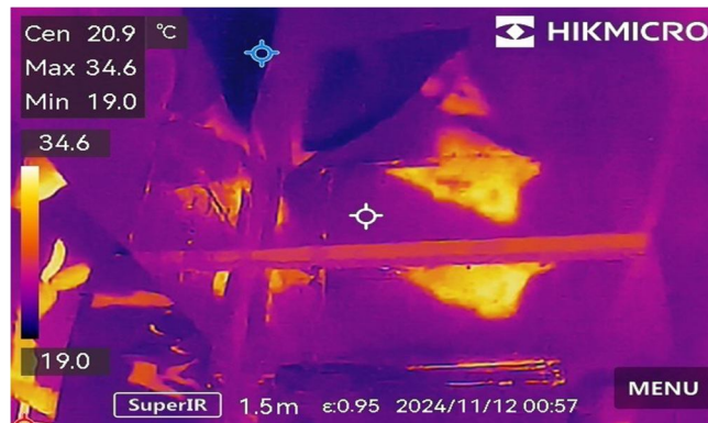
Figure 2 - Thermal Inspection of Ductwork Temperature Variation
