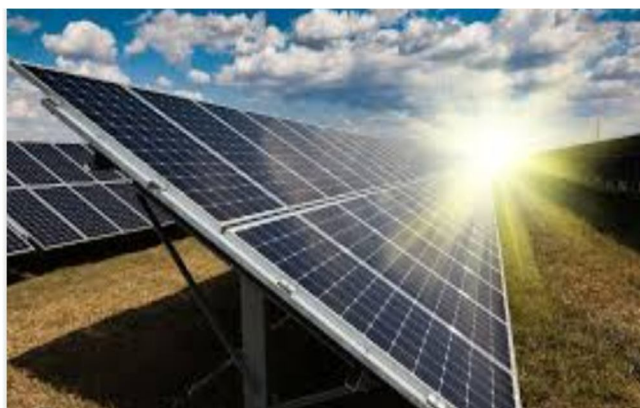
Fig 4.1.6 Solar Panel System
