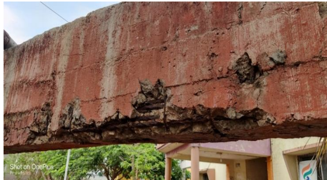
Figure 5 : Exposed and reinforcement at bottom of bracing
