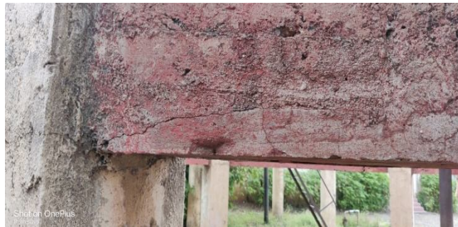
Figure 6 : Cracks in bracing
