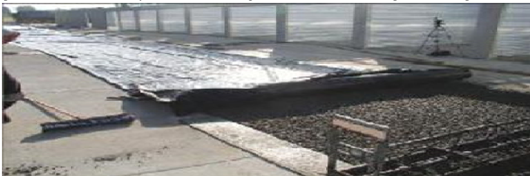
Fig 8 Plastic sheeting should be used to cover the pervious concrete and be installed within a few minutes of consolidation to Prevent moisture loss
