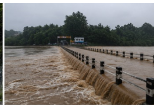
Fig 2: Flooded Bridge During Cloudburst Condition
