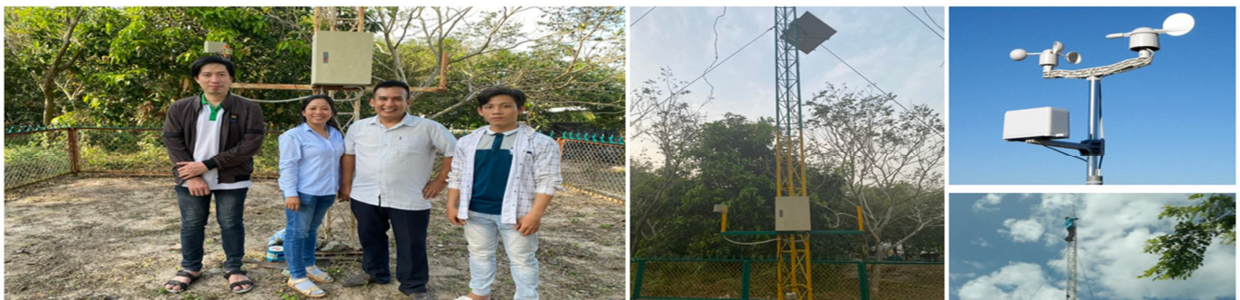
Figure 4: Deployment of the IoT-Based Forest Fire Warning System in An Giang, Vietnam
