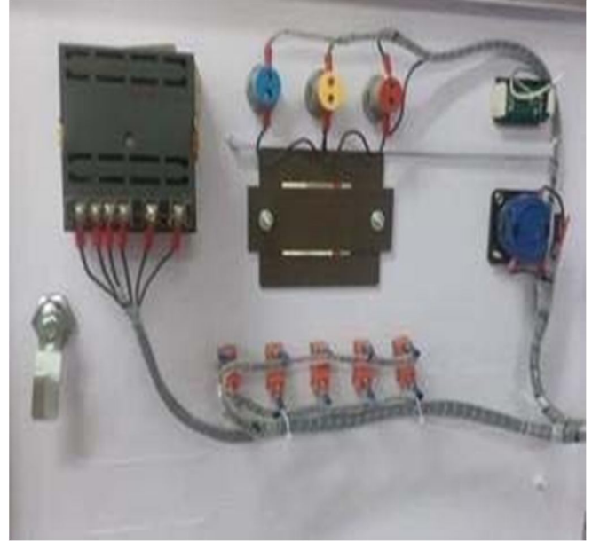
Figure 7(b) - Inside the panel
