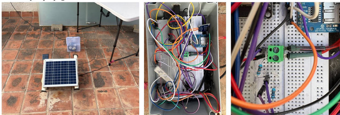
Figure 3: The deployed monitor. (a) The 10 W PV module is shown in its outdoor setting, with the irradiance proxy cell next to it and the enclosure behind it. (b) The enclosure is shown in opened condition, showing the ESP32, the INA219, the microSD module and the load resistors. (c) There is detail of the load network and the sensing connections.
