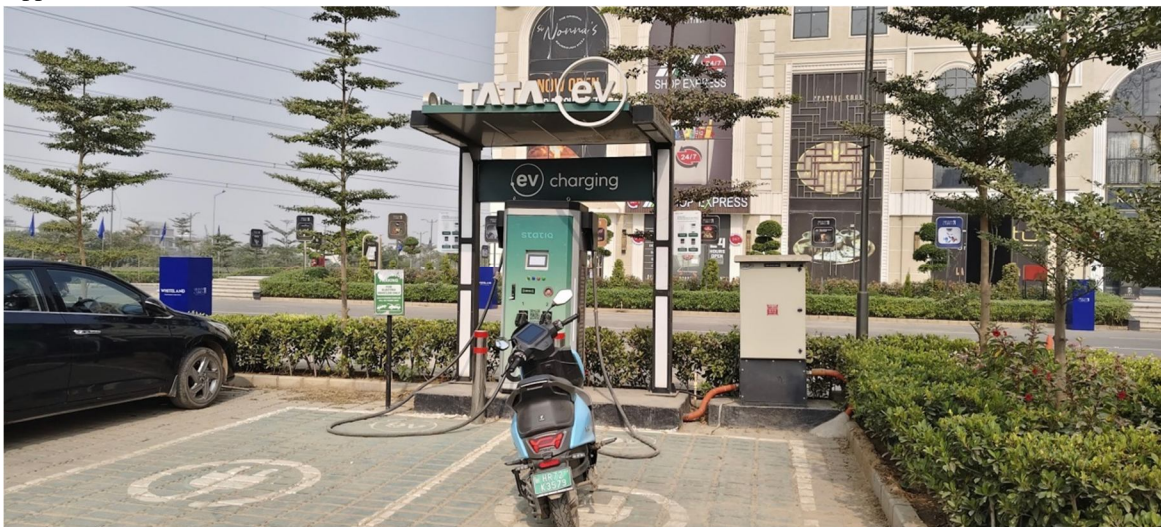
Figure 5: Tata EV charging station accessible via app-based activation but without seating, shelter or rider conveniences, highlighting the mismatch between digital infrastructure and physical user needs during charging wait time
