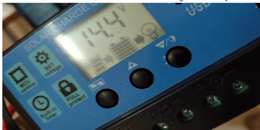
Fig 5.1: Reading from Charge Controller
