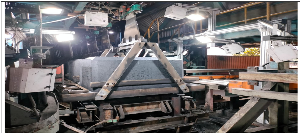
Fig. 11: Anode Visual Monitoring Station.
