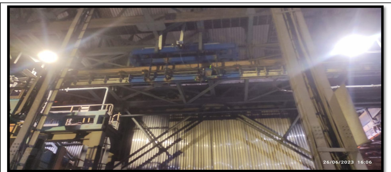
Fig. 10: Online Butt weighing system in P&F Conveyor in ARS.
