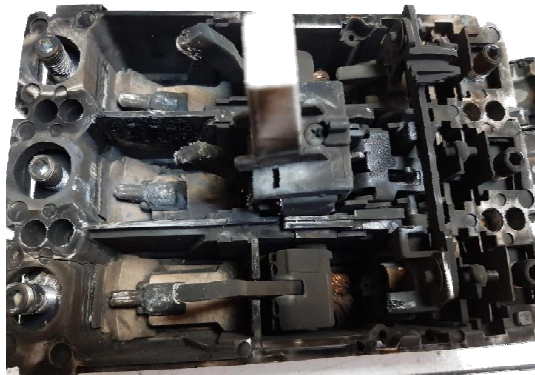
Fig. 6. Damage in Limiter-Equipped Circuit Breakers
