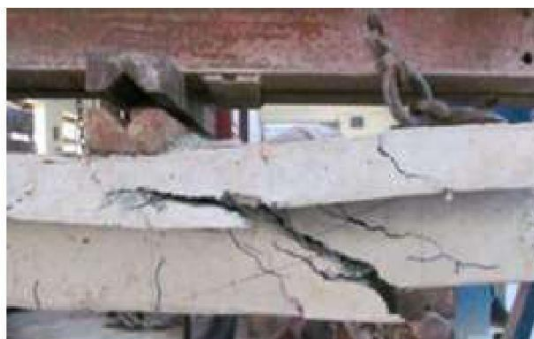
Fig 7 Widened crack at ultimate load
