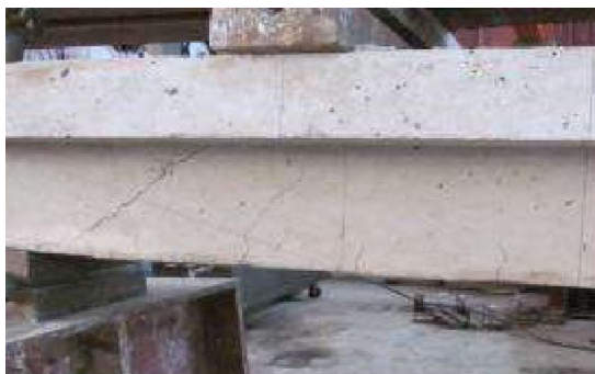
Fig 6 Hair line crack started at 110kN
