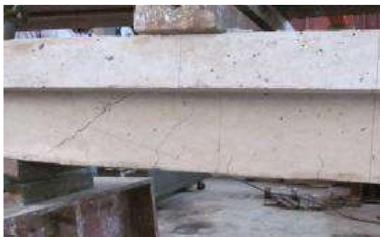
Fig 6 Hair line crack started at 110kN
