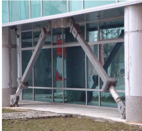
Figure 2. Structure provided with damper
