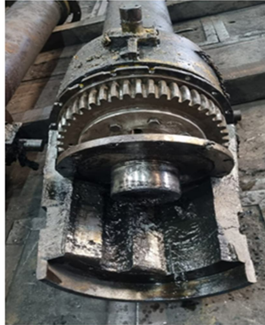
Fig.3 Cracks found nearby wear pad zone
