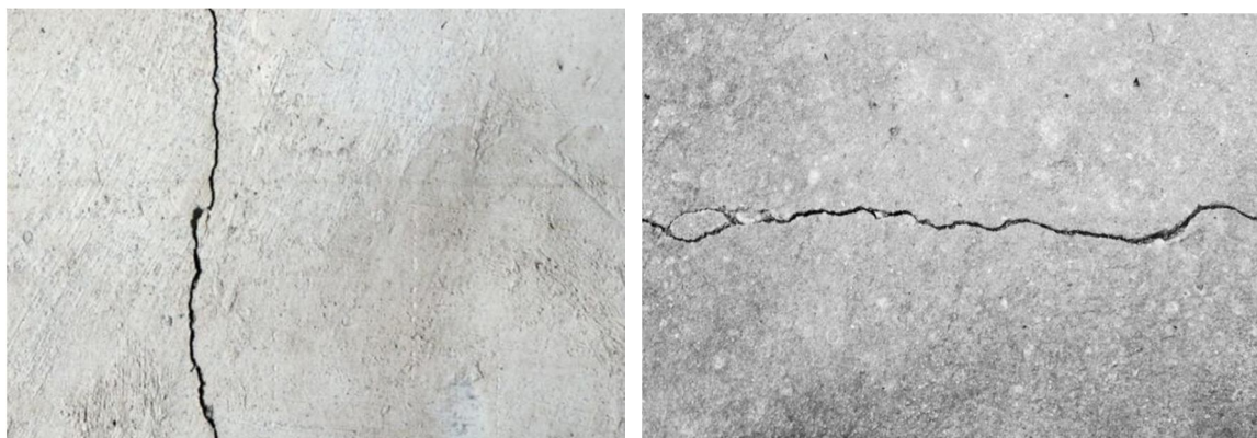
Figure 1. Sample image of crack.
