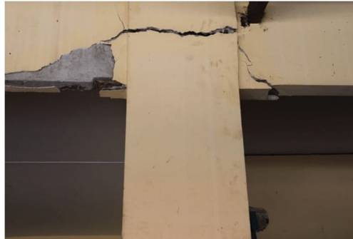
Fig. 3. Site Beam and Column Cracking
