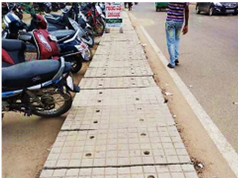
Figure 10:Drain covering as <1m footpath Source: Author
