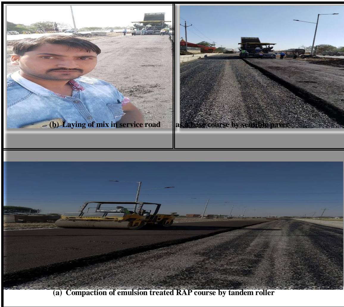
Figure-A) Laying of mix in service road as a base course by sensible paver
