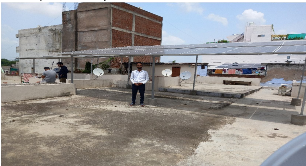
Figure 5. Solar Rooftop Photovoltaic System (RTPV I)
