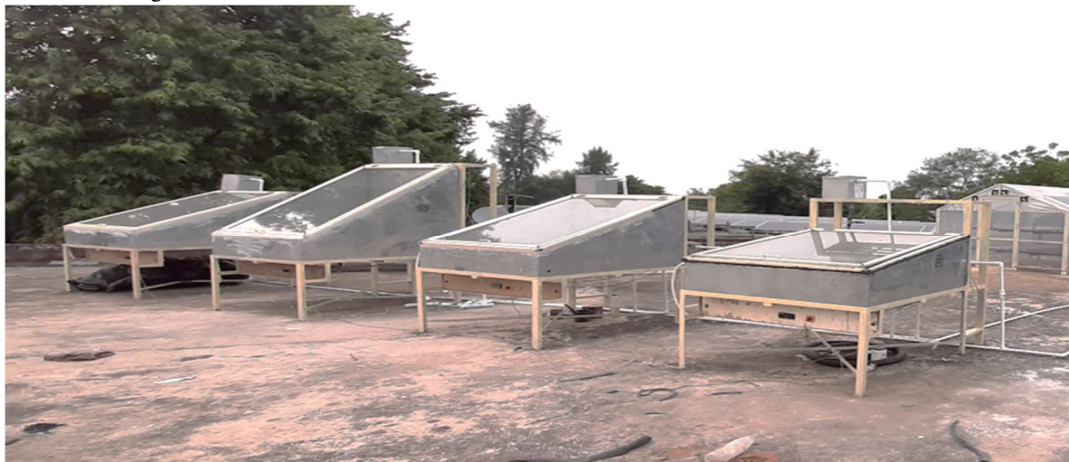
Fig.2 Solar stills installed on MITS Roof
