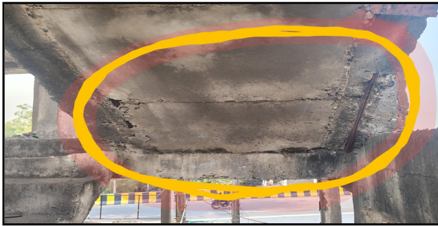
Photo 1) Reinforcement came out of concrete
