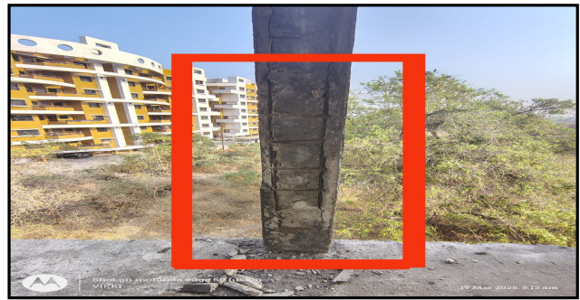
Photo 2) Spalling of concrete from Column
