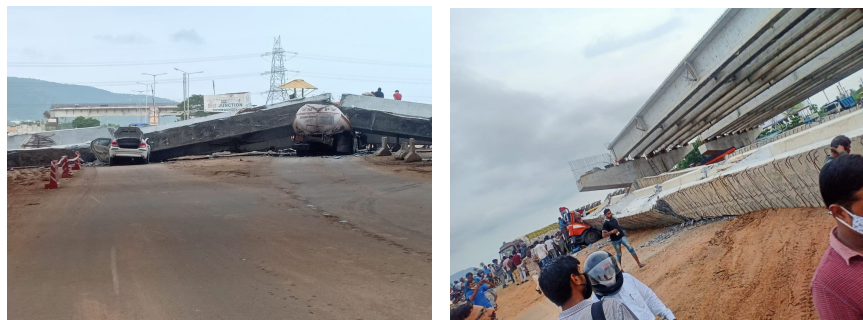
Fig 1.1:- Anakapalli AP NH-16 Flyover Girder Collapse On 6-Jul-2021
