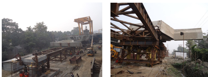
Fig 5.2:- Segment erection failure due to settlement of uncompact bed.
