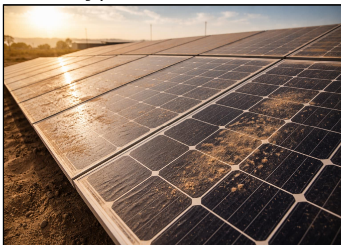
Fig. 1 Shows the Dust-Covered Solar Panels Reducing Photovoltaic Performance
