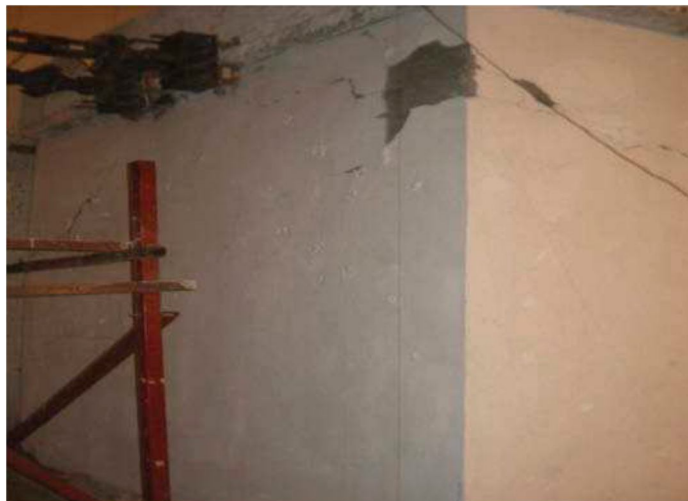
Fig. Falling of plaster observed on retrofitted building.
