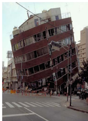
(b) Collapse due to Seismic Torsion
