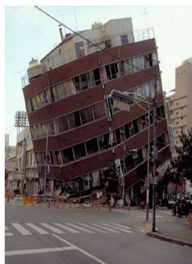
(b) Collapse due to Seismic Torsion
