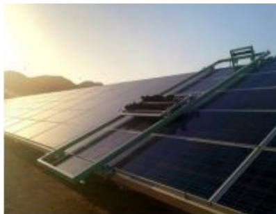
Solar Cleaning System
