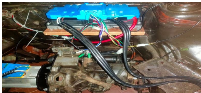
Figure 2. Motor and motor controller
