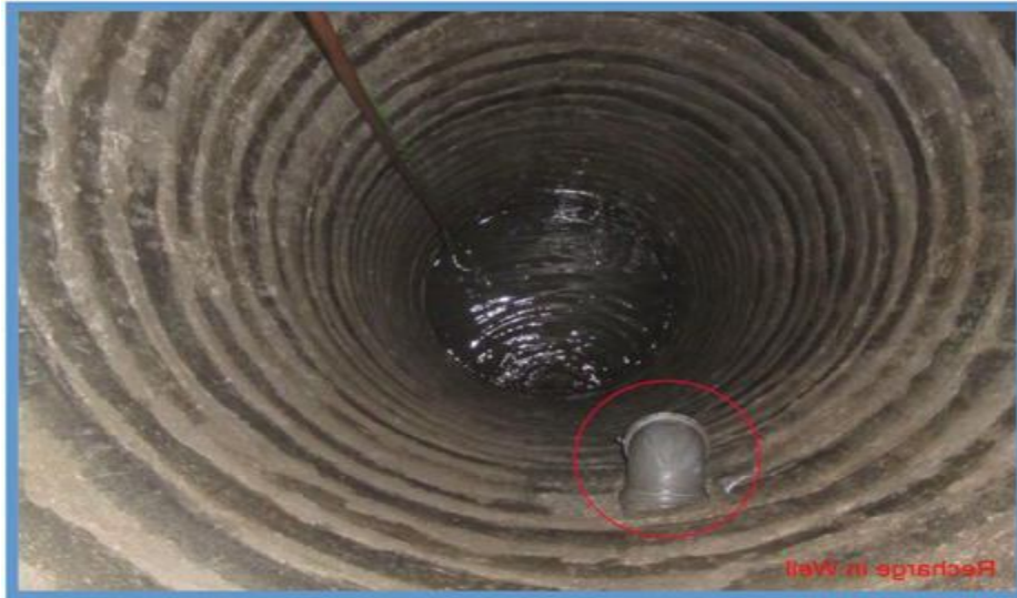
Figure 5 Dug well recharge
