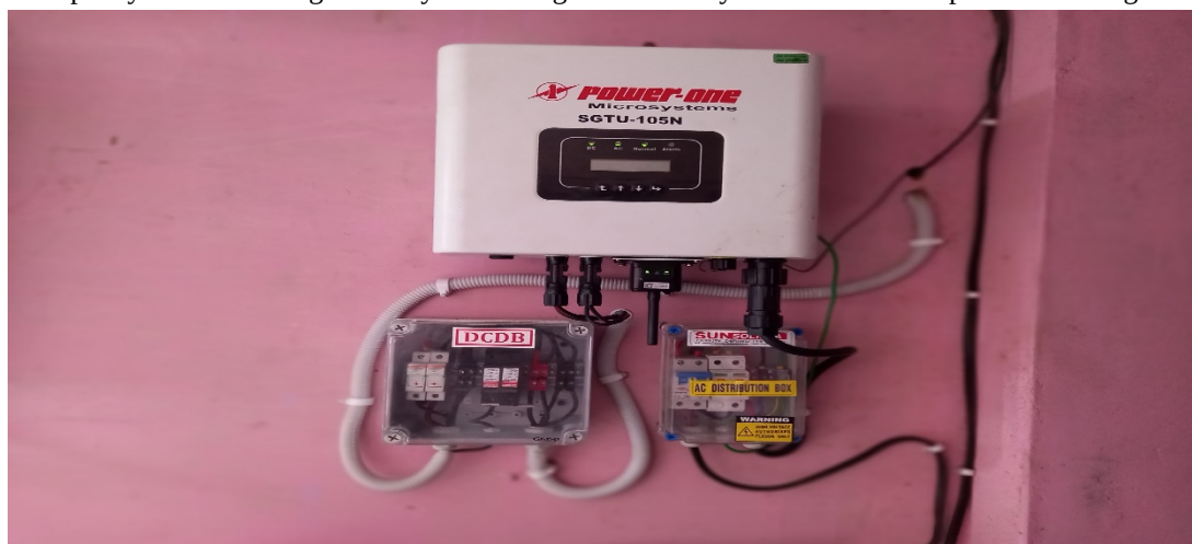
Fig 3 Energy Generation meter.
