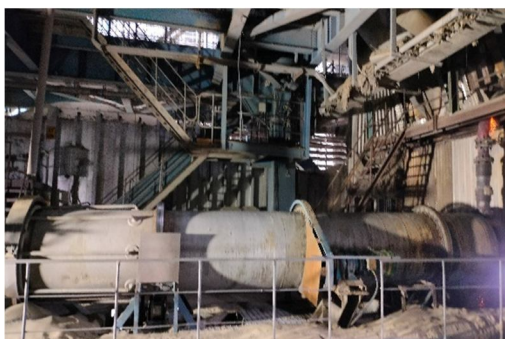
Fig. 1. Water Cooled Slag Cooler of CFBC Boiler
