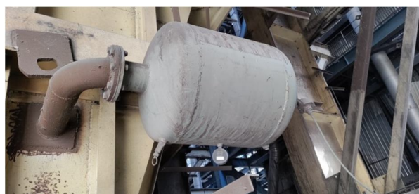
Fig. 3. Air storage Vessel
