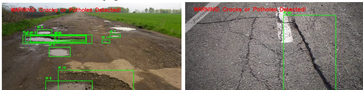
Fig. 2. Detection and tracking of road defects using the trained YOLOv8 model.
