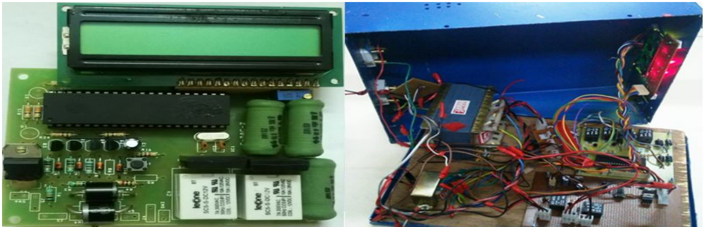
Fig. 5 Open View of power combiner and designed system
