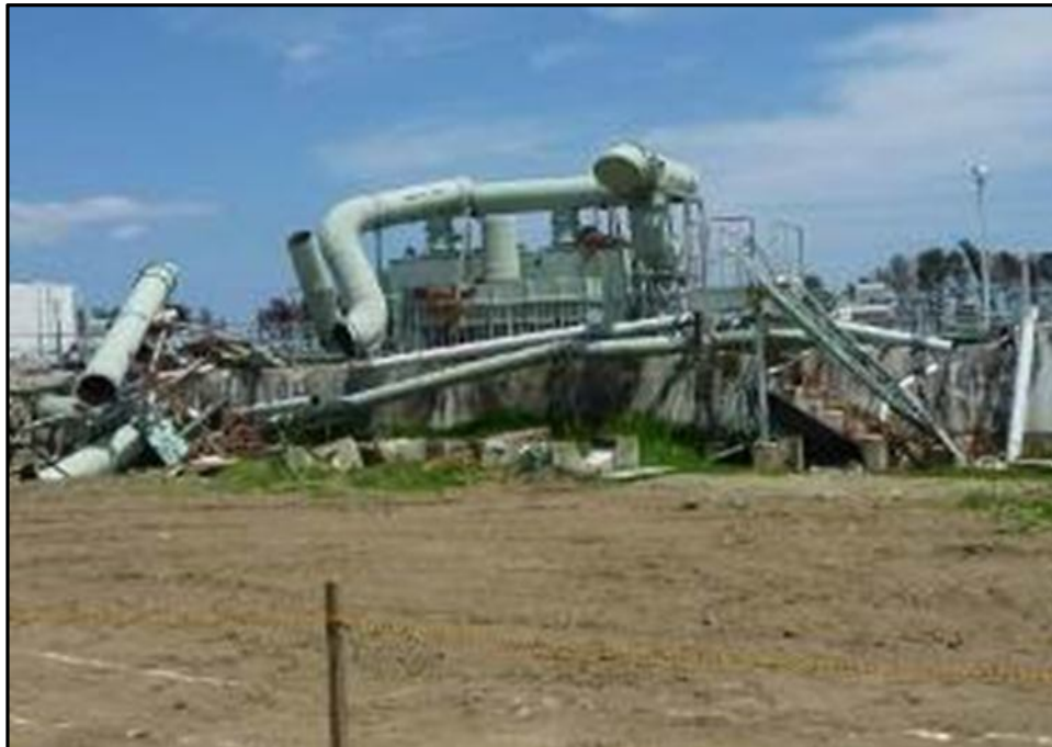
Figure 1: Wastewater Treatment Plant Seriously Damaged by Tohoku Tsunami in the Great East Japan Earthquake 2011.
