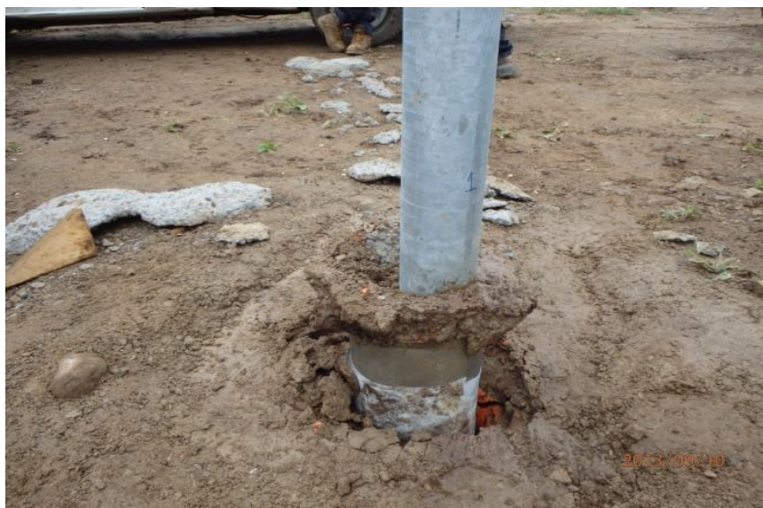
Figure 10. Pile failure in uplift in load testing in soft soils
