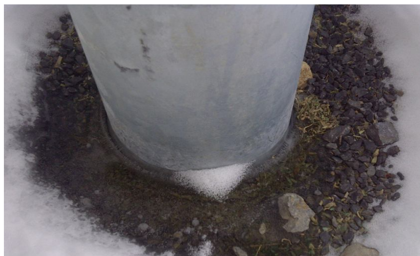
Figure 8. A pile moving out due to frost
