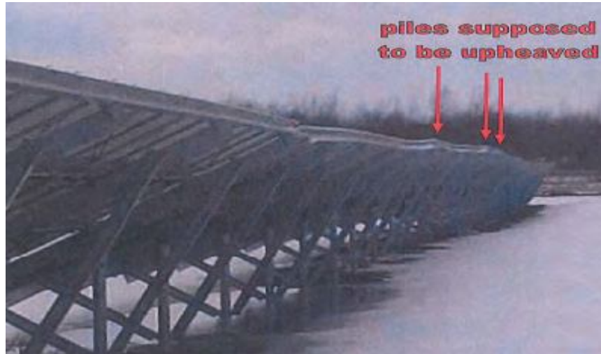
Figure 8. Piles affected by frost showing deformation of the racking
