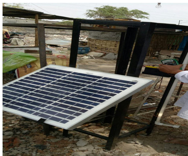
Fig.2: Photographic view of Solar Water Pumping System for Domestic Purpose.
