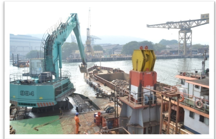
Fig 4.9 Dredging work is in progress by Dharti XXIV at Inner Channel area
