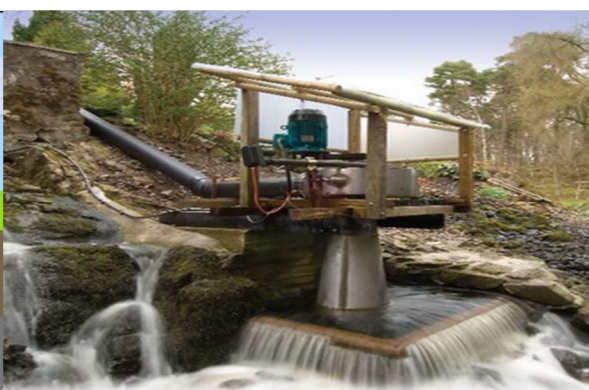
[Fig 12: Power production through SHP Plant]
