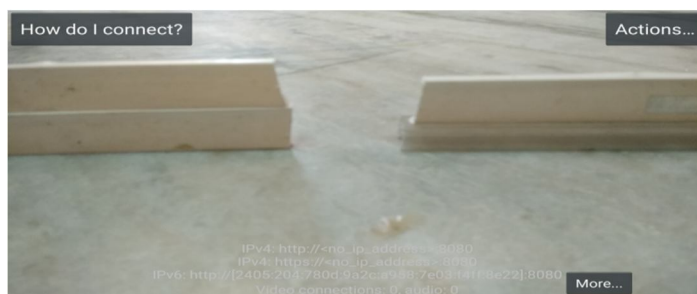
Fig.7 Screenshot of live-video streaming of the crack
