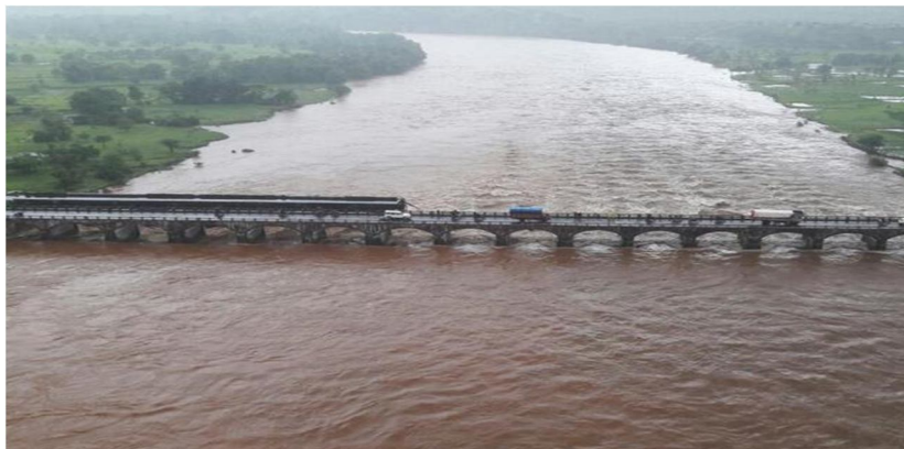
Fig 6. Bridge Collapsed due to heavy rain.
