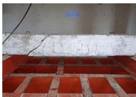
Figure 10 Crack Pattern after Loading
