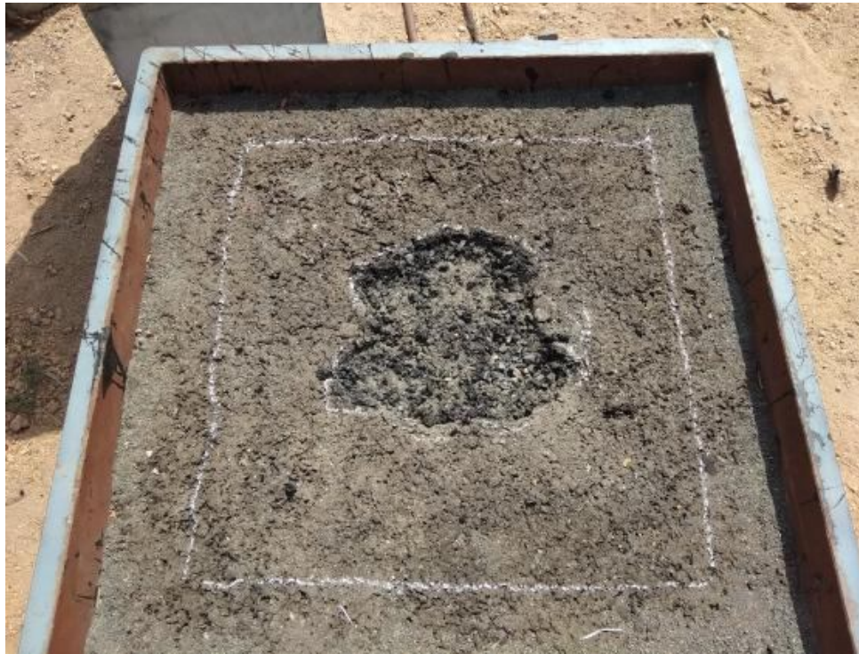
Figure 13 Position of Pothole
