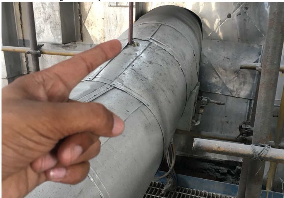
Fig: 6 flue gas sample outlet from economizer
