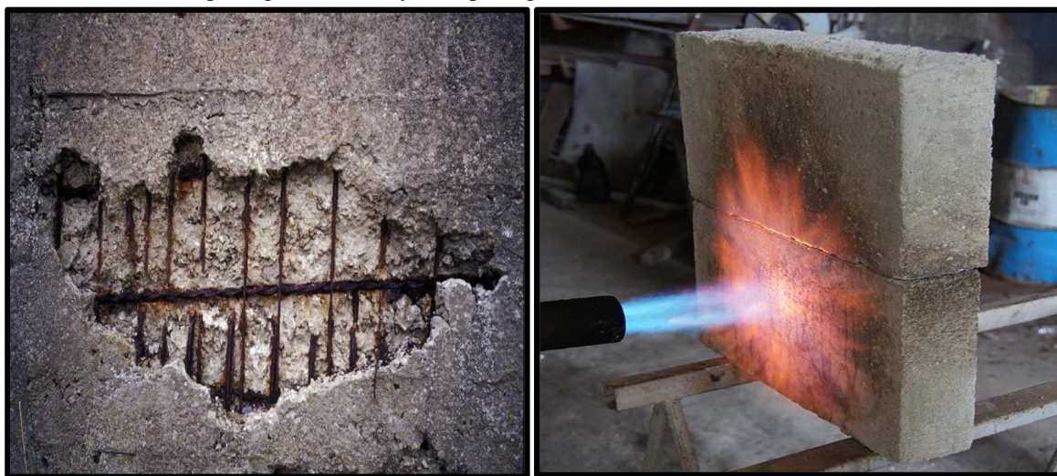
Figure 1. Spalling of concrete
