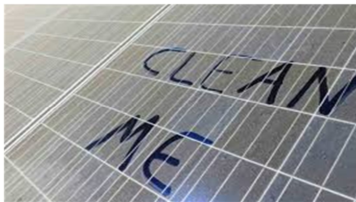
Fig 2: Un-Cleaned Solar Panels
