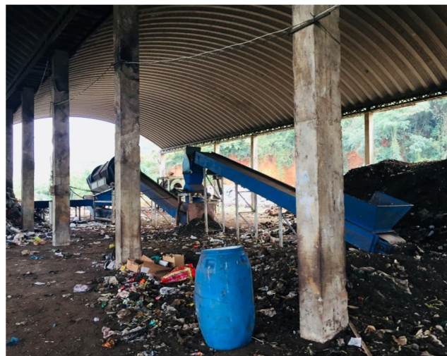
Fig- 5 Segregation machine in Karwar dump yard Shirwad.
