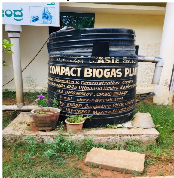
Fig-7 Biogas plant in Science centre karwar.
