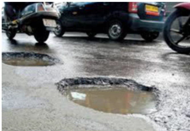
Fig 1. Condition of Indian roads with potholes.
