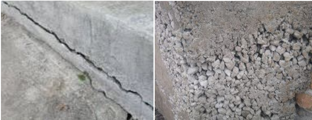
Fig 1: Cracks on concrete surface Fig 2: Honeycombing
