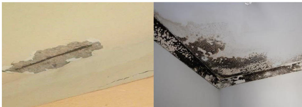
Fig 3: Spalling of Concrete and corrosion of reinforcing bars Fig 4: Moisture Ingress
